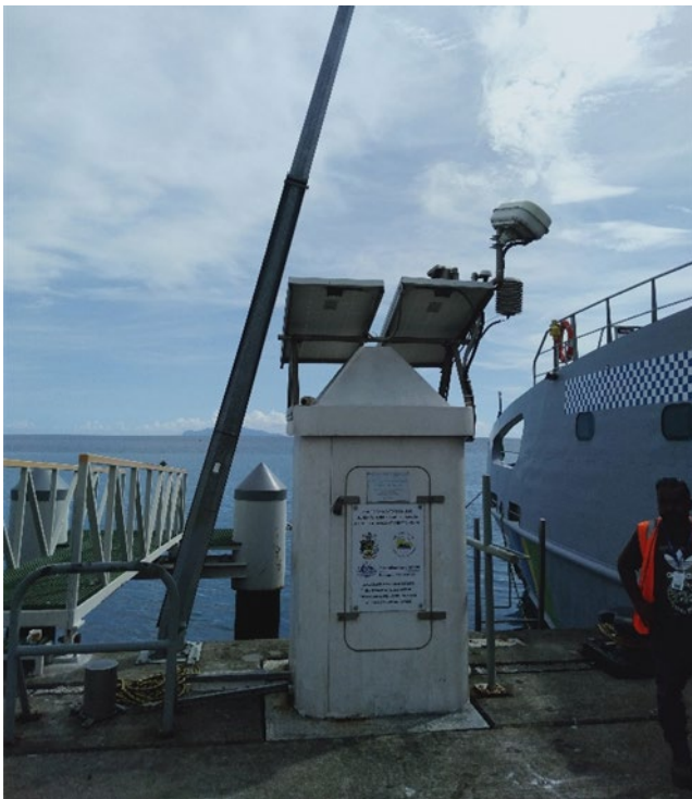
Figure 9 Sea level station at Honiara (anemometer mast is at an angle having been damaged by collision)
